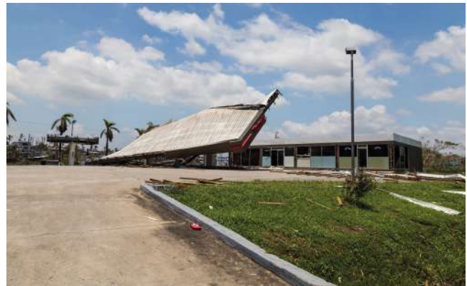
Destruction of petrol station caused by Tropical Cyclone Winston, Island Viti Levu, Fiji.
