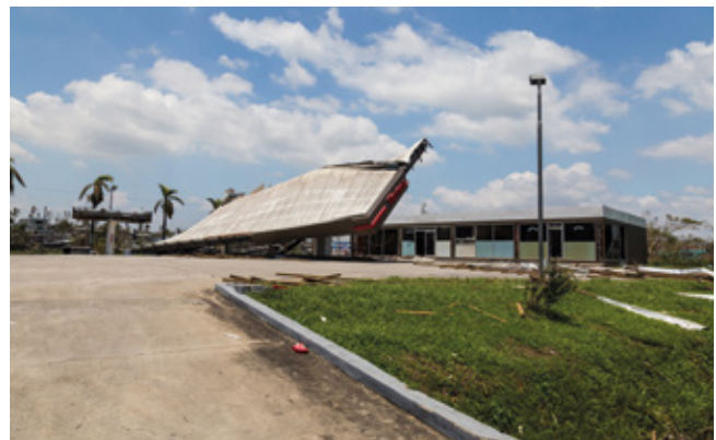
Destruction of petrol station caused by Tropical Cyclone Winston, Island Viti Levu, Fiji.
